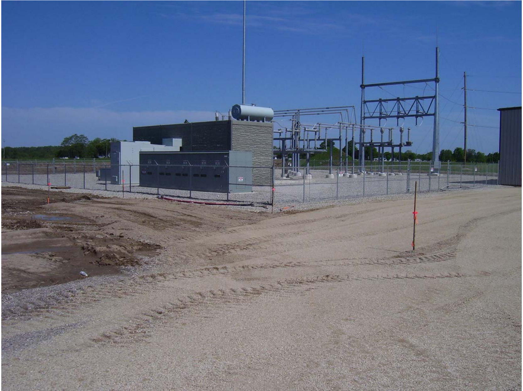
Figure 2-25. Photograph of Representative Substation
